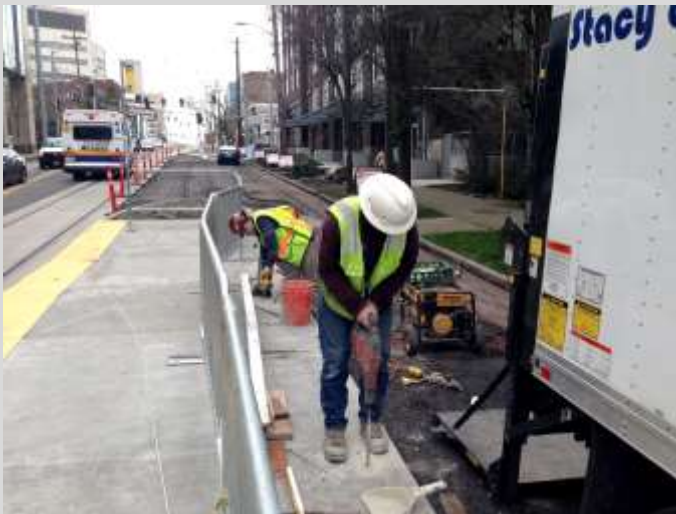
Installing anchor bolts to secure handrails and shelter on the platform at Broadway and Terrace
